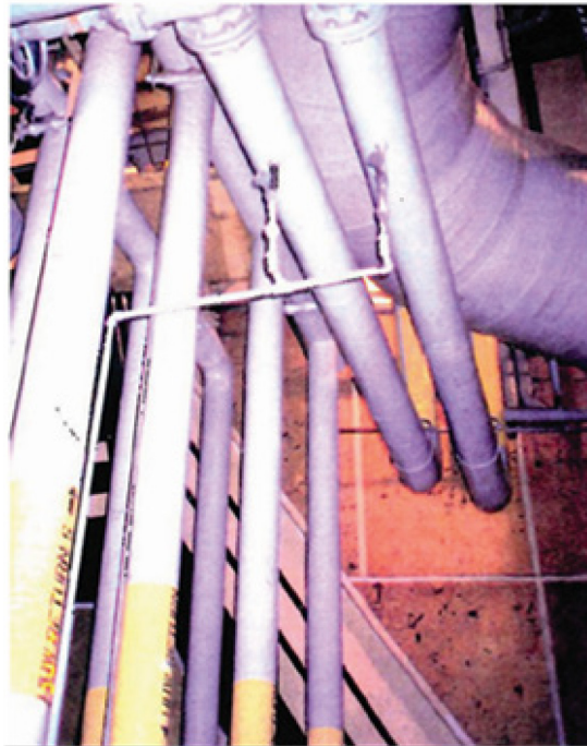
Figure B.10. Detailed view of pipe failure at the industrial facility caused by the Northridge earthquake
