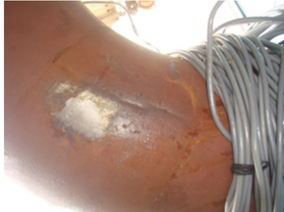
Figure 3.36. Photograph of fatigue-ratcheting failure at the crown of elbow-1 in the CSPS-2 test
