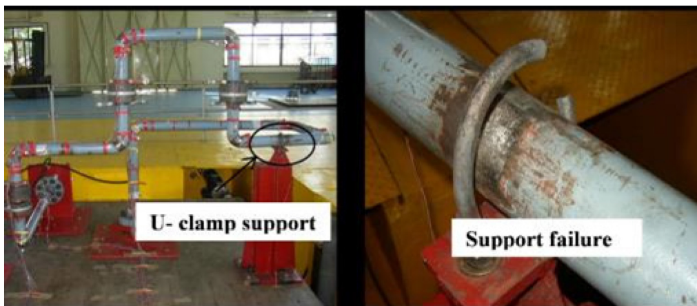
Figure B.26. Failure of the U-clamp support during a shake table test on a piping system
