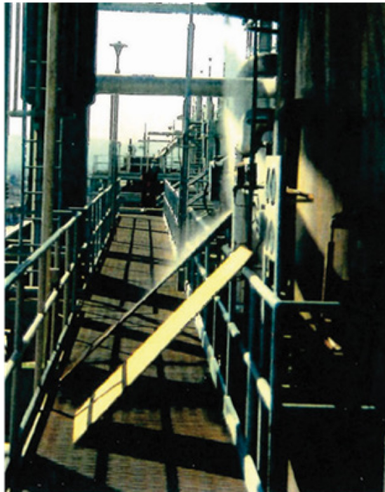
Figure B.15. View of the leaking corroded elbow in a condensate line as a consequence of the Northridge earthquake
