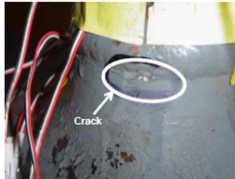
Figure 3.25. Photograph of a wall crack at the weld location of tee and pipe
