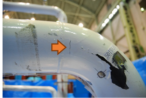
(b) Fatigue failure at a wall thinning elbow, close to the pipe end (Elbow1 of AP3_C31, NIED_Test#02)
