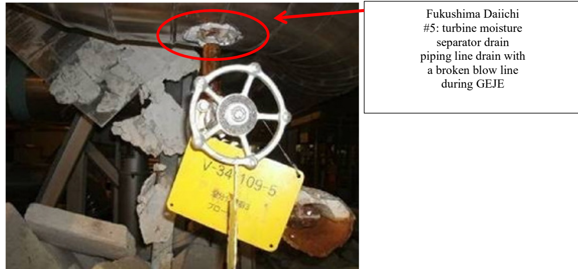
Figure B.24. View of damage to the piping support section in a thermal power plant
