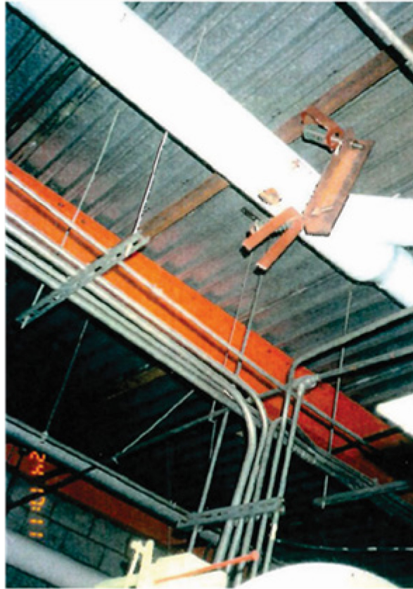
Figure B.9. Detailed view of pipe support failure at the industrial facility caused by the Northridge earthquake
