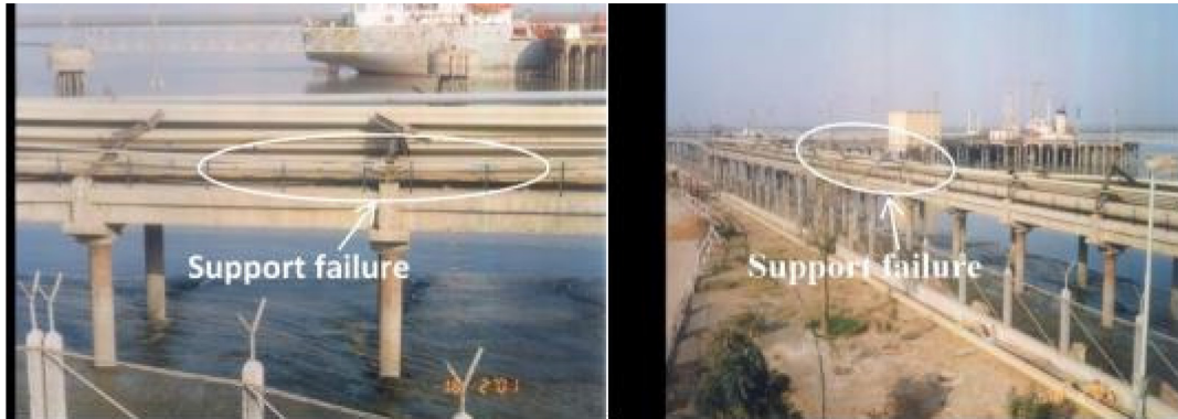
Figure B.27. Failure of piping supports during the Bhuj earthquake, India, 2001 (Mw 7.7)
