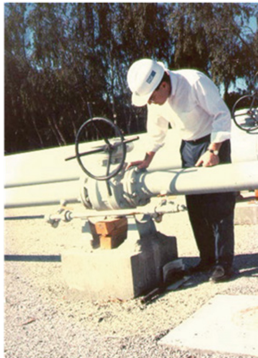
Figure B.17. Soil liquefaction caused the support saddle to drop nearly 12 in. (25 mm) in the Loma Prieta earthquake
