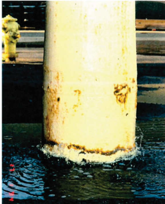
Figure B.14. View of the leaking corroded inlet riser to the cooling tower at ground level due to the Northridge earthquake
