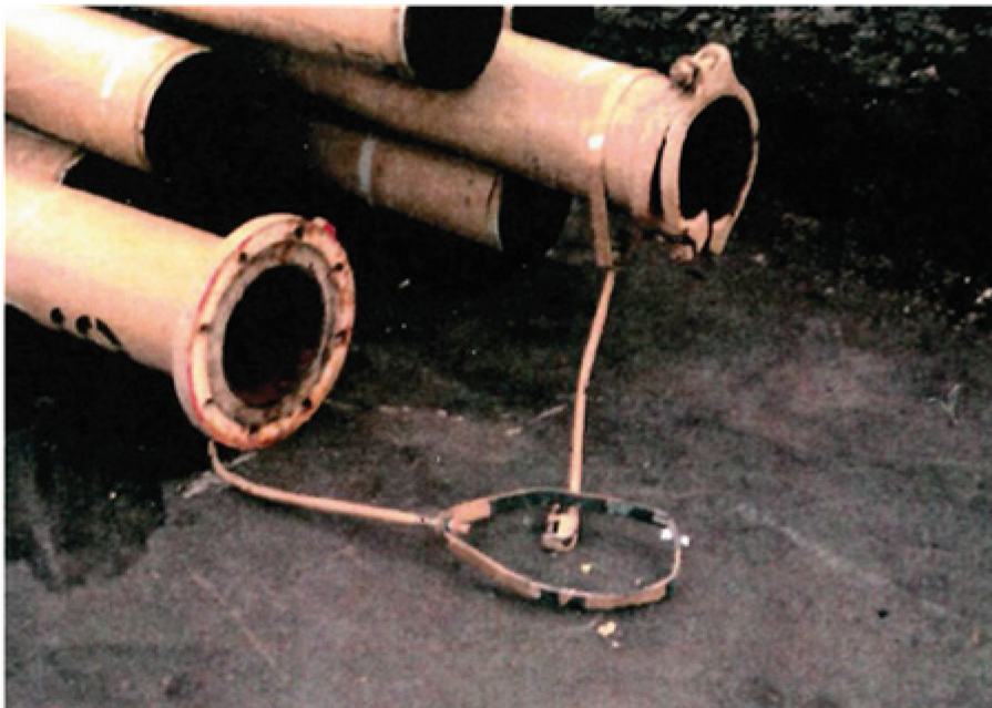
Figure B.13. Fire protection pipes affected by the Northridge earthquake
