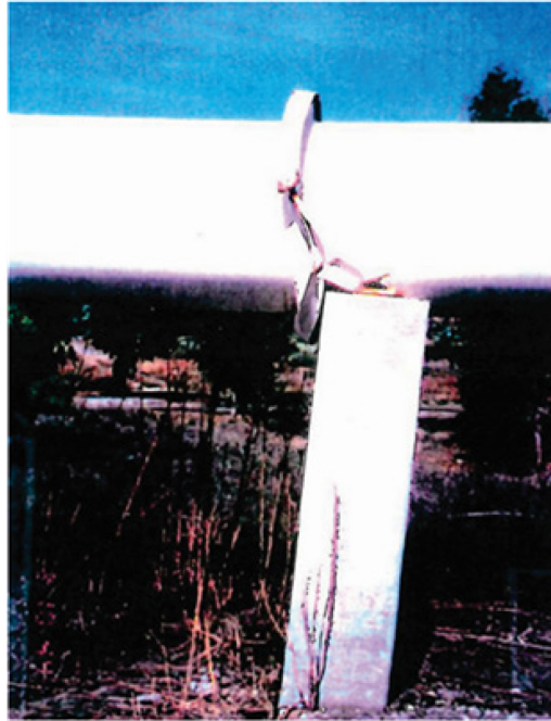
Figure B.16. Pipe support failure from ground failure produced by the Northridge earthquake
