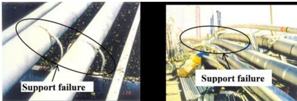
Figure B.28. Failure of piping supports during the Kobe earthquake, Japan 1995 (Mw 7.0)
