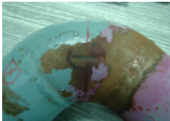
Figure 3.28. Photograph of the dent at the crown location of elbow-1
